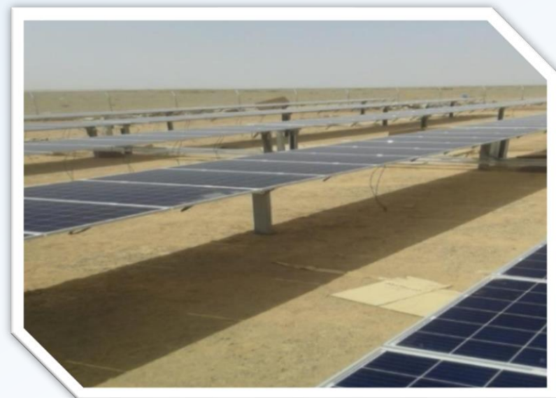
10 MW PV power plant (Qom Province, Iran)
