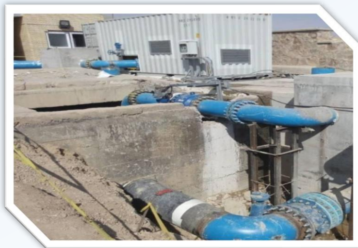
3 MW capacity Small Hydropower (Semnan Province, Iran)
